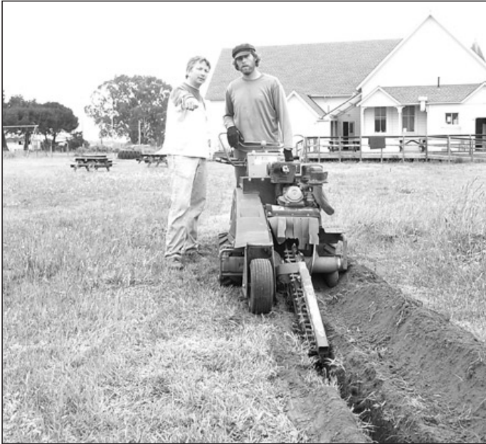
Tom Brown and Paul Garvin trenching for the garden water and electrical hook-ups. July 2008
